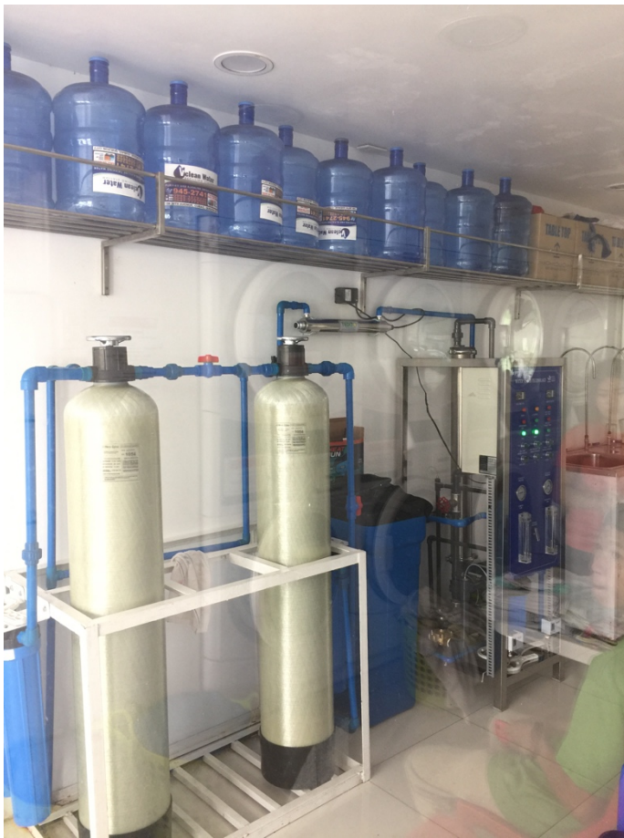
A water-treating facility near my apartment. Thankfully, water proved not to be the root of my issue – this would've made life in QC quite difficult (and expensive).
